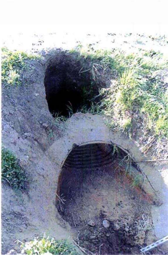
Corrugated Culvert Pipe with serious structural deterioration prior to lining.
